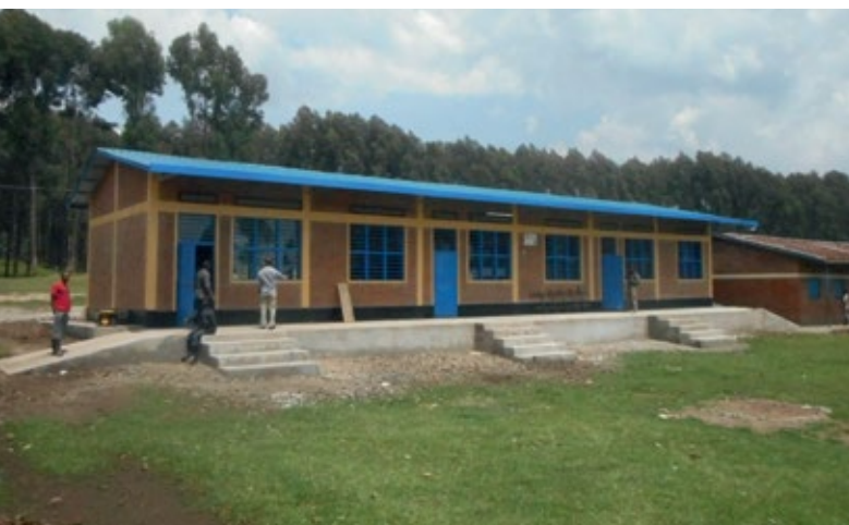
A building at the Kampanga school in Musanze District on which a PV system will be installed © Municipality of Enkenbach-Alsenborn
