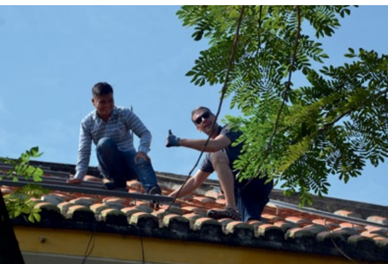
February 2018 saw the installation of the photovoltaic system in Hoi An, which was supported by Engagement Global/the Service Agency. © Lothar Andert
