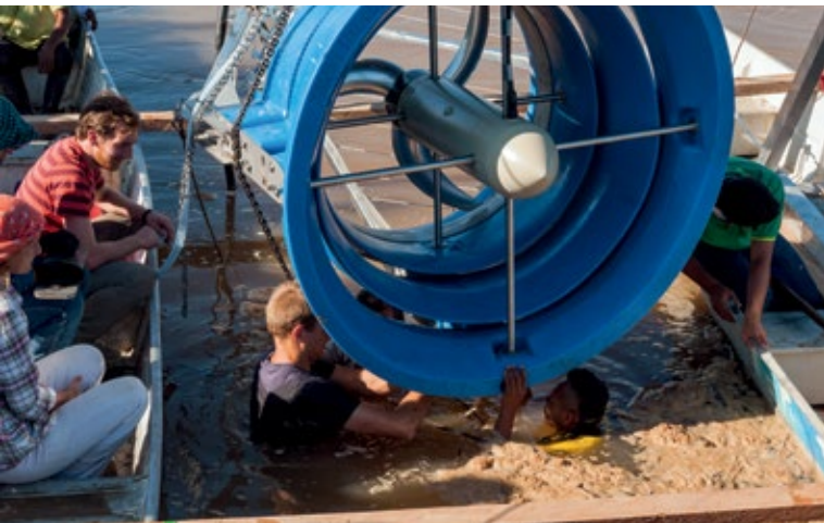
The project in full flow – actors from Schondorf and Puerto Leguizamo installing the turbine imported from Germany. In combination with solar cells it is being used to power the newly procured electric boat. © Stefanie Windhausen
