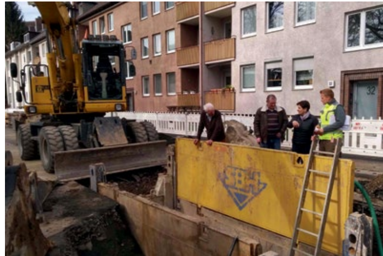
Visiting a construction site in Kassel, organised by the Municipality of Gudensberg. The participants from Schtschyrez are looking at some underground construction work. There are plans to lay a sewer in Schtschyrez in the same way. © Stadt Gudensberg
