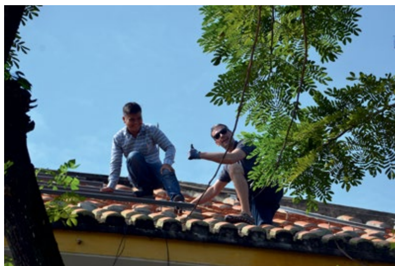
Up on the roof: Two engineers installing a photovoltaic system at the tourist information office in Hoi An in Viet Nam. Written cooperation agreements between the municipalities of Hoi An and Wernigerode provided the firm foundations on which this project was built. © Lothar Andert
